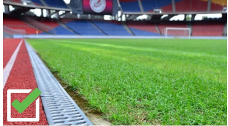
Proper drainage cover
