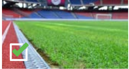
Proper drainage cover
